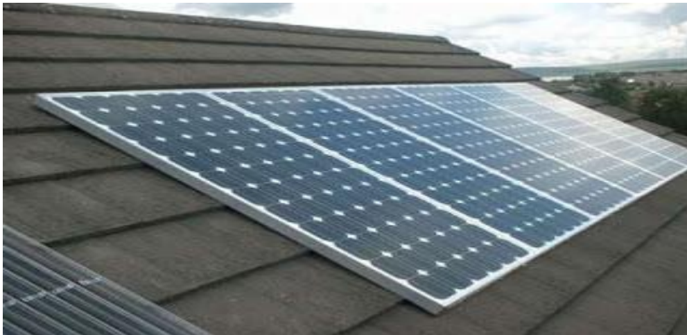
Figure (2.1) Mounted Solar Panel at Rooftop
